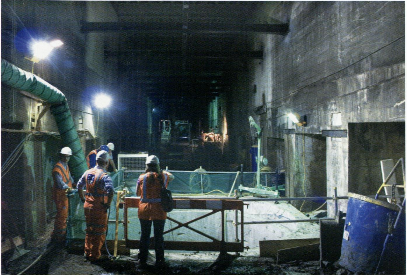
The grout shaft under construction in the floor of the Kingsway tunnel in London during the construction of Crossrail. After completion the Grade II listed tunnel will be returned to its original condition. Photo Ian Mansfield
